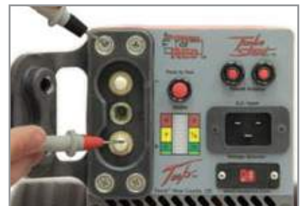
3. Place the negative probe to the fastener screw on the dc Receptacle. Move the positive probe to the dc positive post. Multimeter should read 0 Volts.
