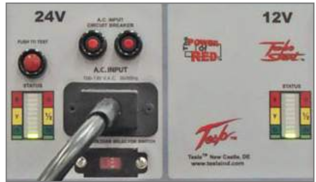
Figure 3.12.2 - AC Power Connected with LEDs Illuminated
