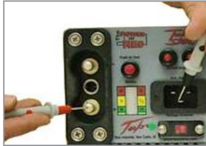
2. Place the negative probe on the ac ground post and the positive probe to the dc positive post. Multimeter should read greater than 10 MΩ.
