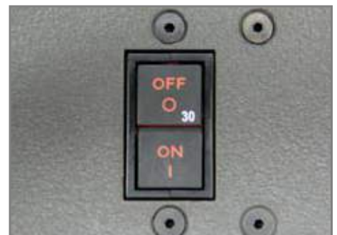
Figure 3.16.7 Circuit Breaker ON
