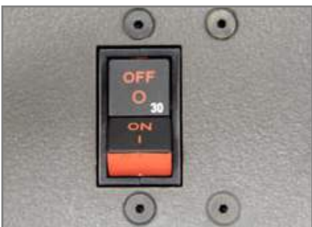
Figure 3.16.5 Circuit Breaker OFF
