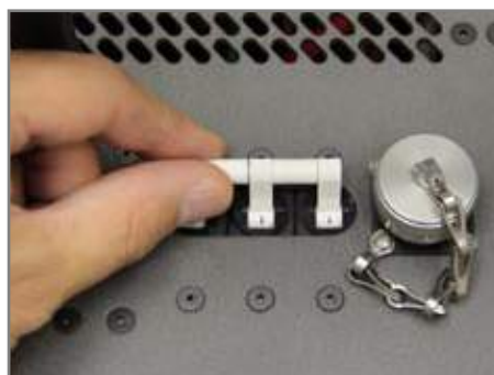
Figure 3.16.6 Switching Circuit Breaker ON
