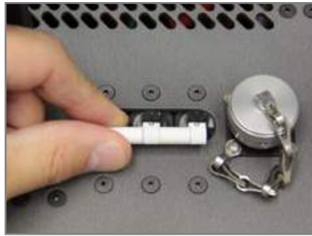
Figure 3.16.2 Switching Circuit Breaker OFF
