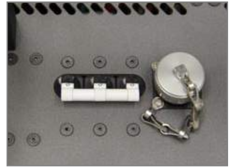
Figure 3.16.3 Circuit Breaker OFF
