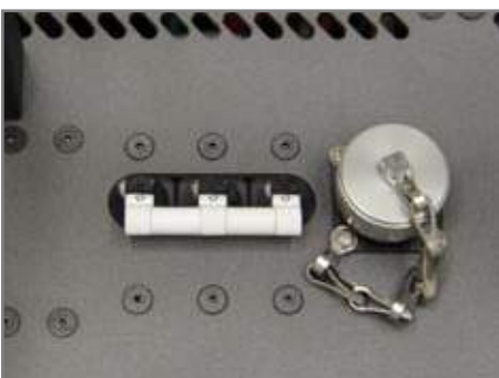
Figure 3.16.5 Circuit Breaker OFF
