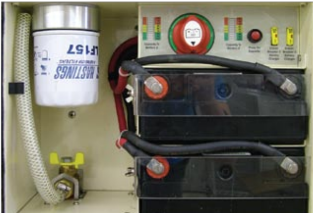
Figure 13: Oil Filter, 12 Volt Batteries, and Battery Selector Control Panel
