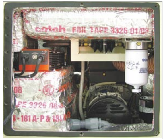
Left Engine Access Panel - Fuel Filter, Generator, Oil Cooler, and 2 internal Battery Chargers
