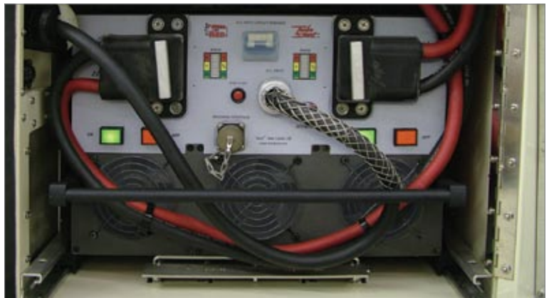
Dual DC Receptacles and Tesla™ Ground Power Unit
