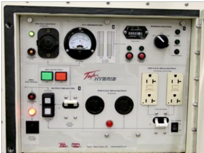
Main Electrical Control Panel
