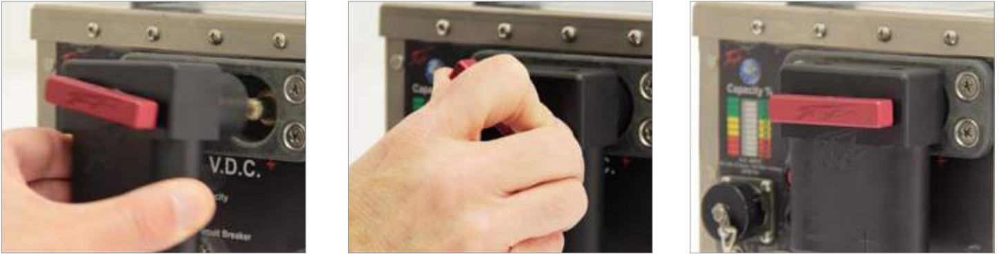
Figure 3.10.1 Attaching dc power cable to TI58D MPU-24
