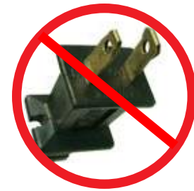
Figure 1.3.3 – Improper Ground Plug with No Grounding Pin
