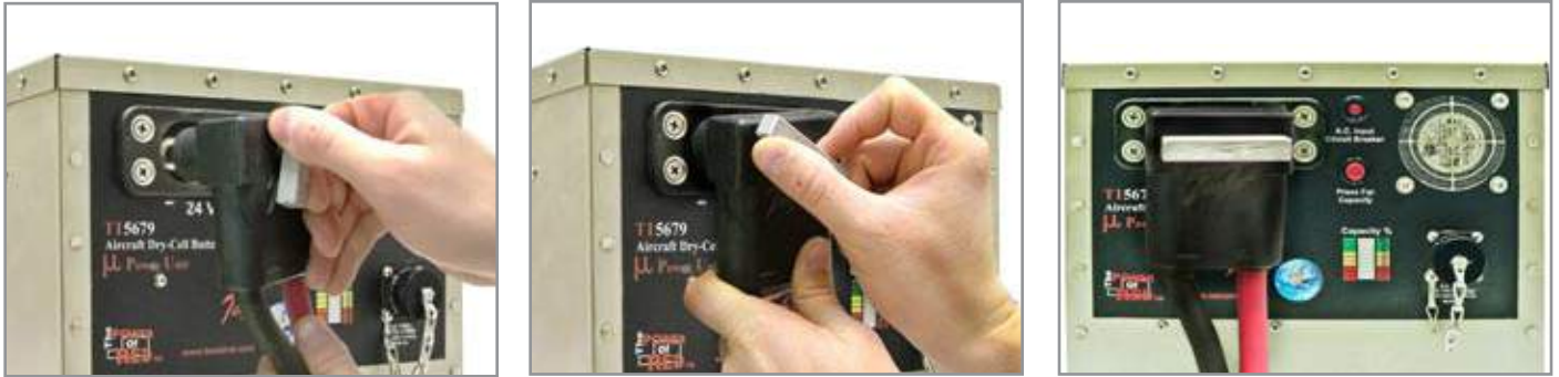
Figure 3.10.1 Attaching dc power cable to TI5679 MPU-24
