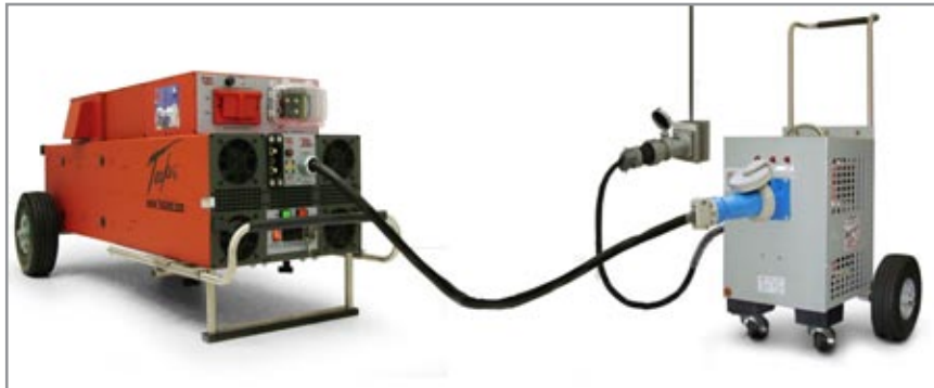
Figure 6.4.1 Transformer connected to GPU
