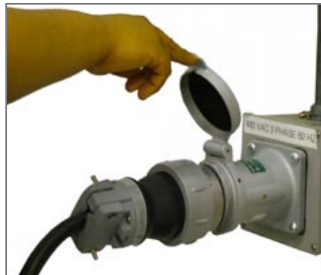
Figure 4.2.2 480 VAC cable plugged in.
