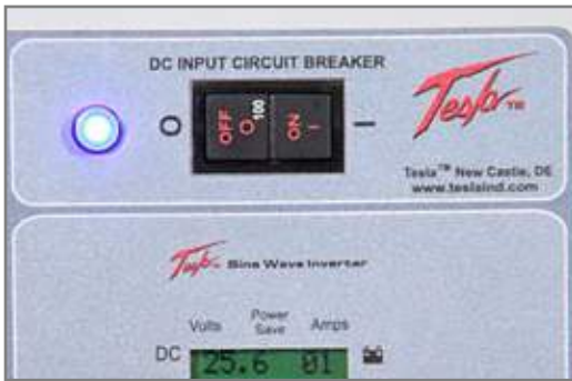
6.3.1 60Hz AC Inverter Power set to "ON" position (LED illuminated)
