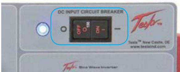
Figure 3.14.1 TI3000 GPU-24-INV-1800 DC Input circuit breaker in “on” position (outlined in blue)
